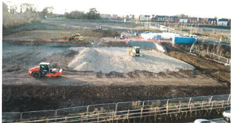
The above photo shows ongoing ground works which we have scheduled for the months of January, February, March.
